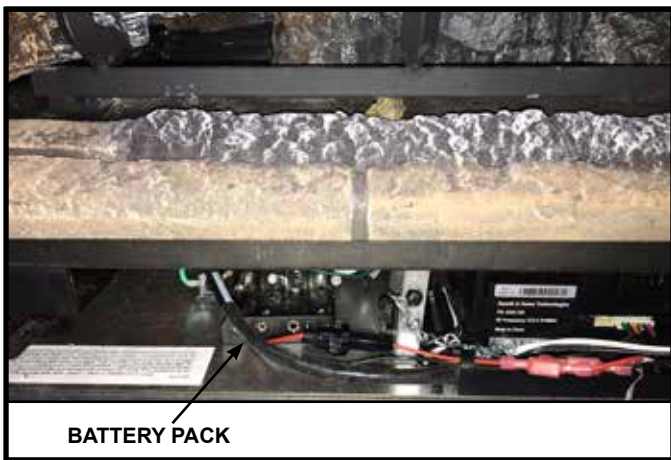
Figure 3.8 Battery Pack Installed
