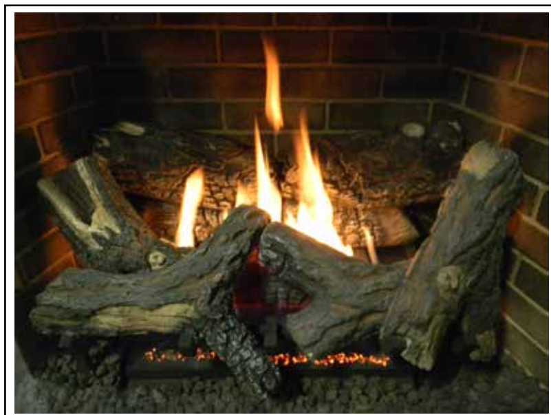
Figure 34C - Burner Flame Appearance
